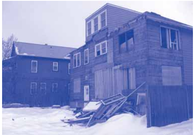
The porch and ramp were removed to make way for an addition.
