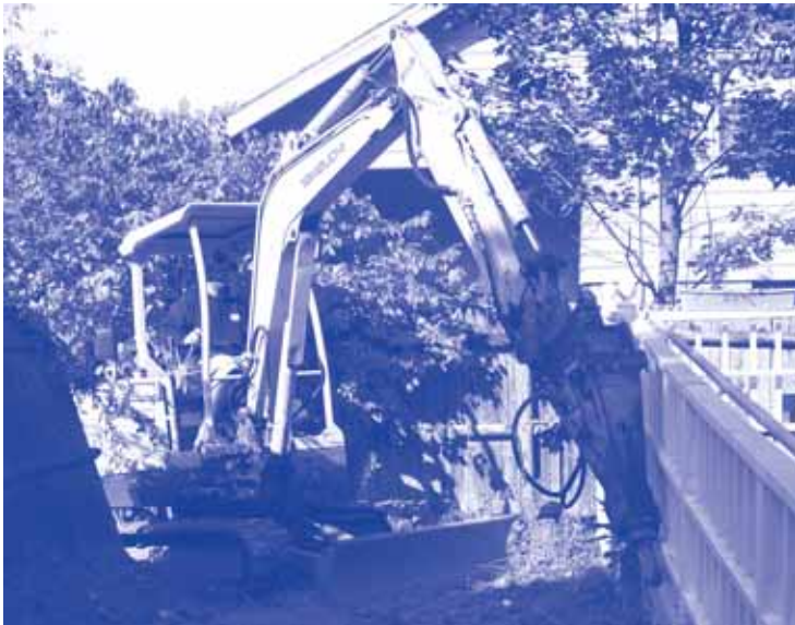
S+H Construction moves in equipment. Chan Mock Architects are also involved with the project.
