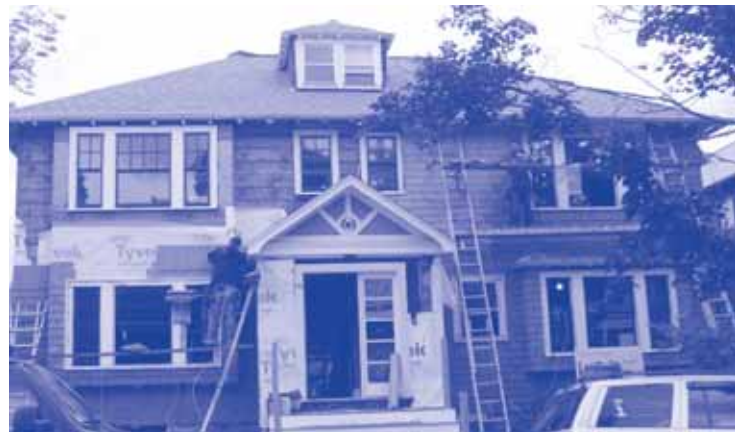
Chilton House now has high efficiency, double pane, low-E coated, argon filled windows. New siding is also being installed.
